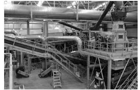
Percolators at WSN recycling centre. Photo: WSN Environmental Solutions
